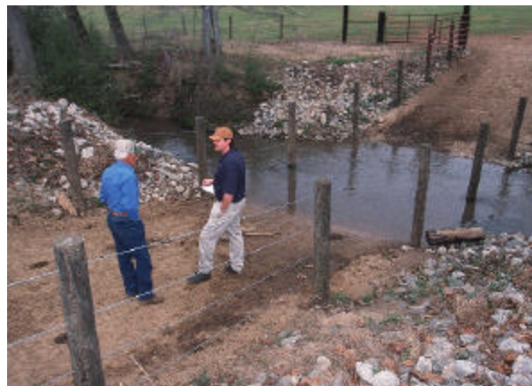
Stream Crossing Protection Can Reduce Erosion and Cattle Time Spent in the Stream
