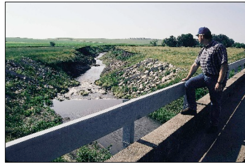
Rip rap installed on a stream bank helps control livestock access and minimize erosion. Photo by Lynn Betts, NRCS.
