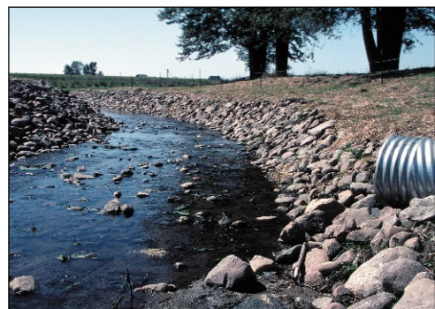
This stream bank has been stabilized and protected from erosion by rip rap. Photo courtesy of the NRCS.
