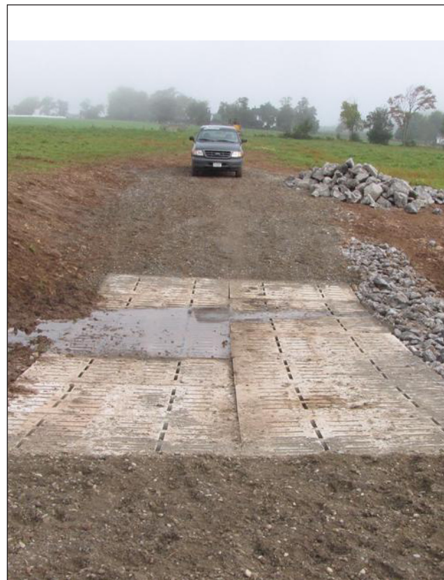
Figure 20. Hardened crossing points constructed of geotextile fabric, concrete panels, and fine gravel to facilitate cattle movement across specific points in the stream. Photo courtesy of Chenago County Soil and Water Conservation District.
