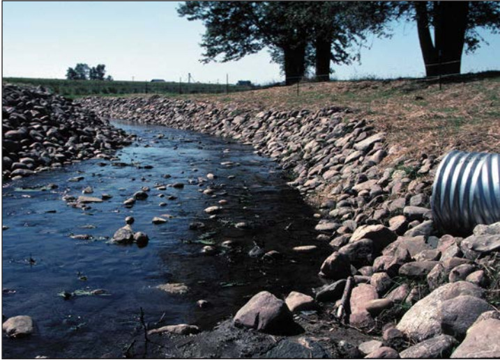
Figure 22. This stream bank has been stabilized from erosion with rip-rap. Photo courtesy of the USDA-NRCS.
